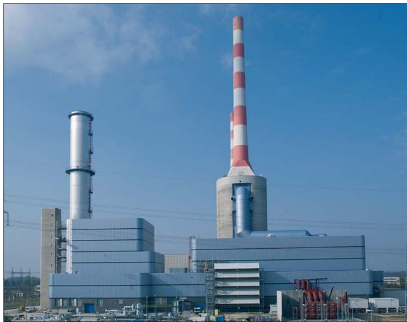
Power plant Irsching: stationary gas turbines have gained 40 %, in combination with steam turbines in combined cycles they reach slightly more than 60 % – admirable, not only for the engineer
